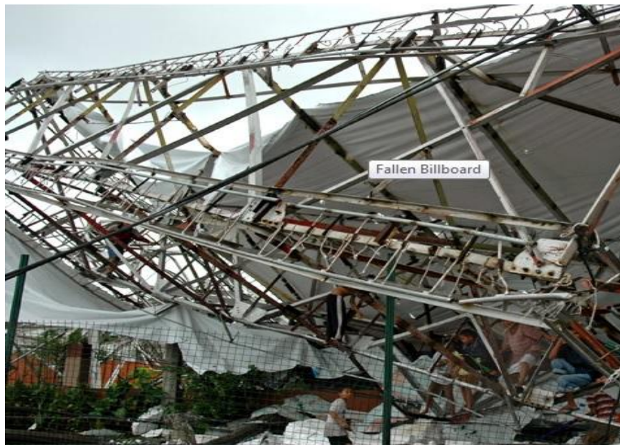
Figure 7: Billboard Structure (inadequate gusset plate)
