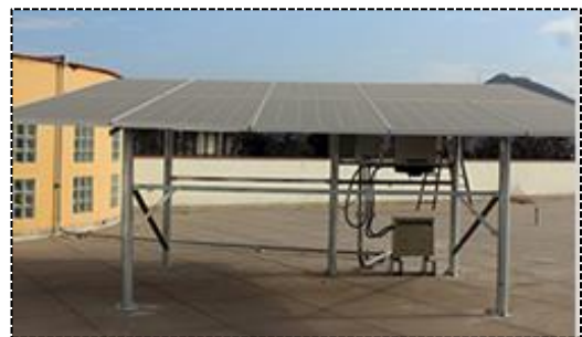
Fig. 3. A 3.25-kWp Solar PV System
