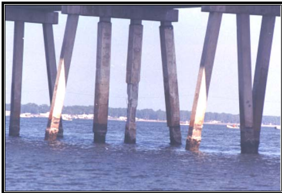
Figure 1: One of the Bryant Patton Bridges Displaying Reinforced Concrete Piles with Significant Corrosion Induced Damage - Florida (reproduced from Concorr, Inc).
