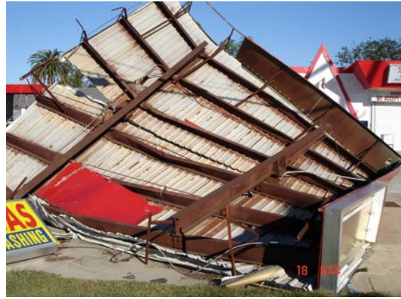
Figure 10b. Road 90 and Wright, New Orleans area. Purlings hang from the beams. (Photograph taken on November 18)
