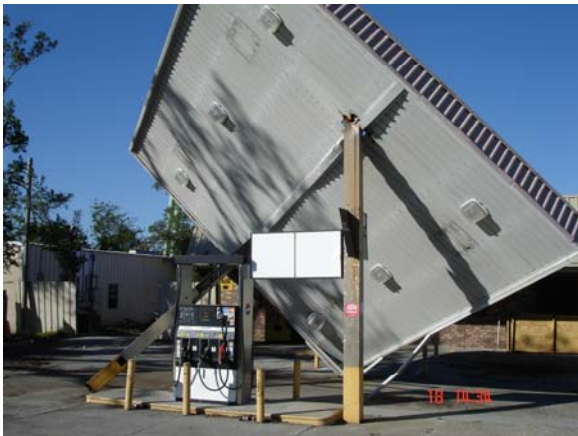
Figure 6a. St. Bernard, LA. One of the columns failed due to plasticity. (Photograph taken on November 18).
