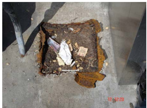
Figure 4c. Chevron gas station in Vidor, TX (Photograph taken on October 12).
