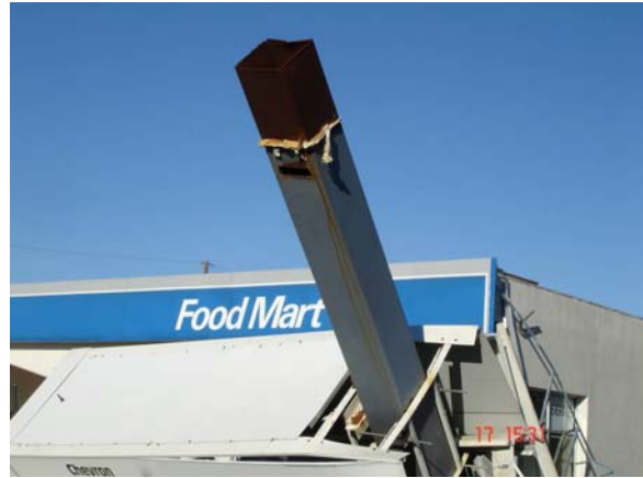
Figure 8b. Chevron gas station in Meraux, LA. The columns did not have connection with the roof. (Photograph taken on November 17).
