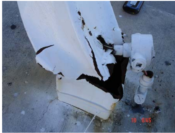
Figure 10c. Road 90 and Wright, New Orleans area. Fracture at the base. (Photograph taken on November 18).
