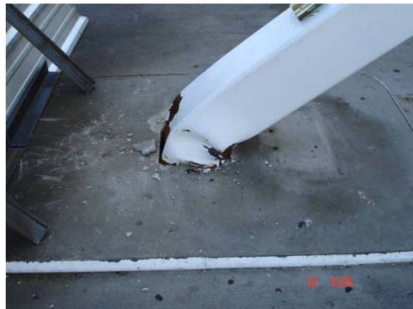
Figure 3b. Exxon Gas Station, Hillerbrandt, TX. Plastic hinges formed at the base of the columns. (Photograph taken on October 12).
