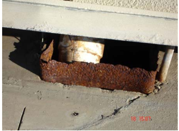
Figure 5b. Road 39, Chalmette, LA. Evidence of corrosion at the base of the columns. (Photograph taken on November 18).
