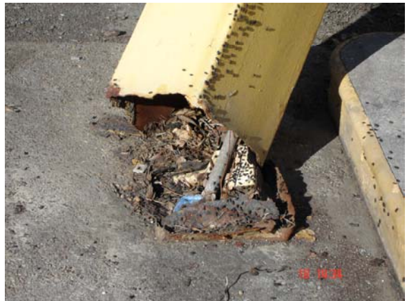
Figure 6b. St. Bernard, LA. One of the columns had extensive corrosion at the base. (Photograph taken on November 18).
