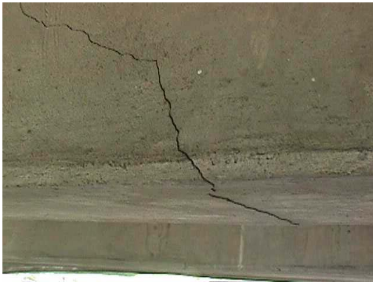
Figure 4: Crack in Exterior Girder
