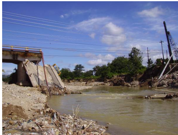
Figure 3: Damages to Madre Vieja Bridge.
