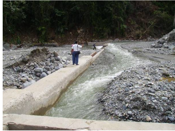
Figure 8: Water Supply Intake Damages
